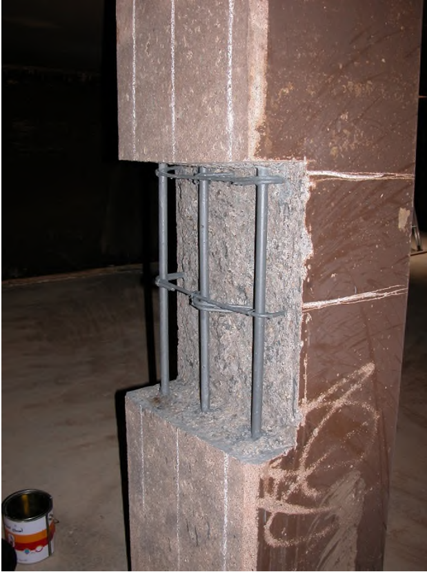
Figure 3 - Shows grey colour of properly prepared steel
